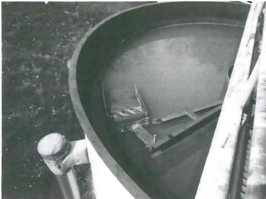
P5070004.JPG – Skimmer arm missing a rubber squeegee in the second primary settling tank. Scum build-up in trough (in need of cleaning) and solids build-up on ramp.
