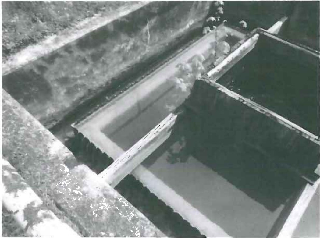
P5070012.JPG – Solids build-up behind weir in final effluent chamber
