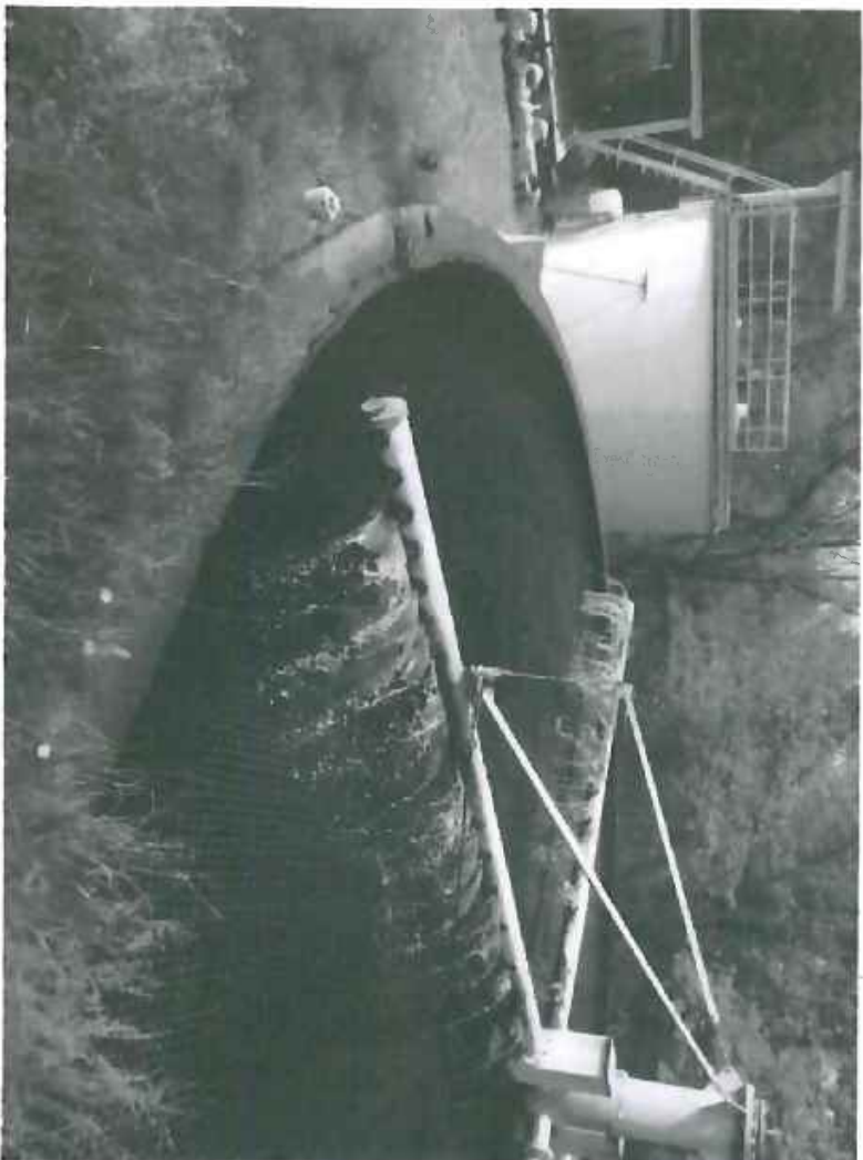
P5070007.JPG – Trickling filter with clogged nozzle
