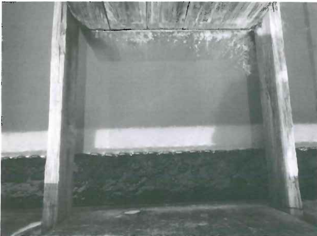
P5070014.JPG – Close up of solids build-up in final effluent chamber
