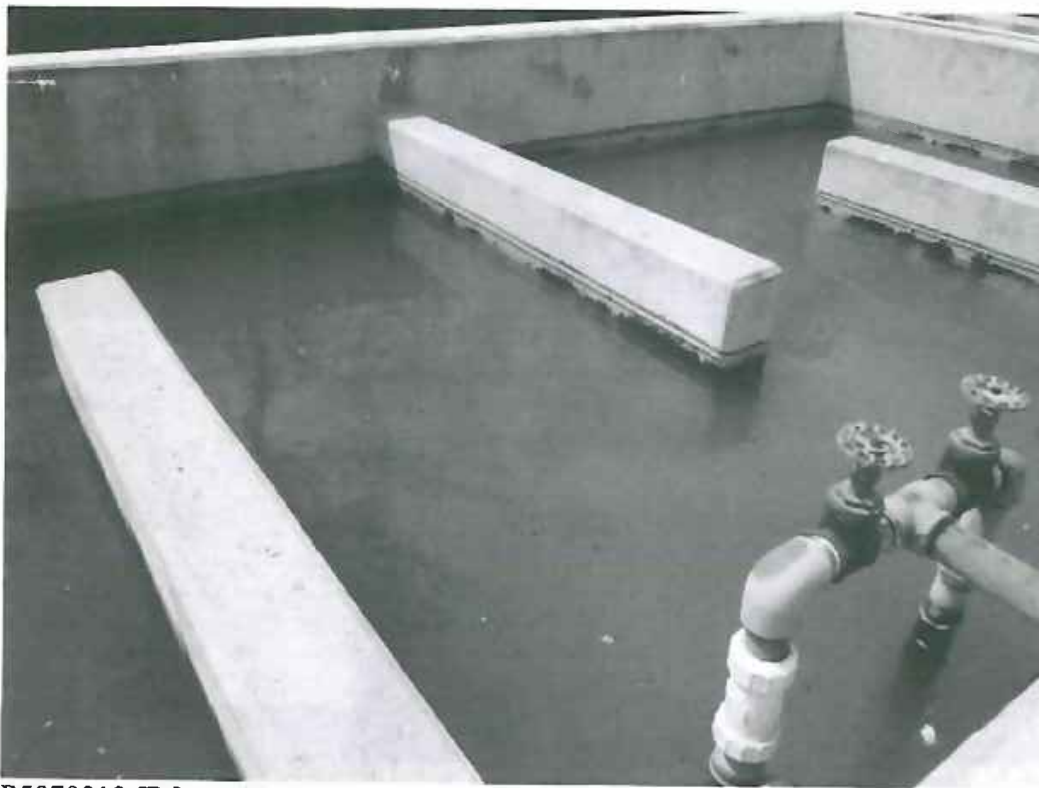
P5070019.JPG – Chlorine contact tank
