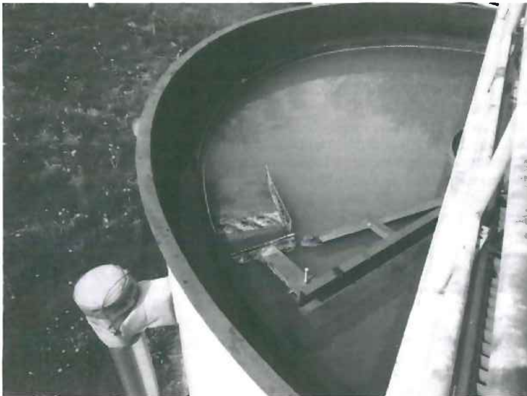
P5070004.JPG – Skimmer arm missing a rubber squeegee in the second primary settling tank. Scum build-up in trough (in need of cleaning) and solids build-up on ramp.
