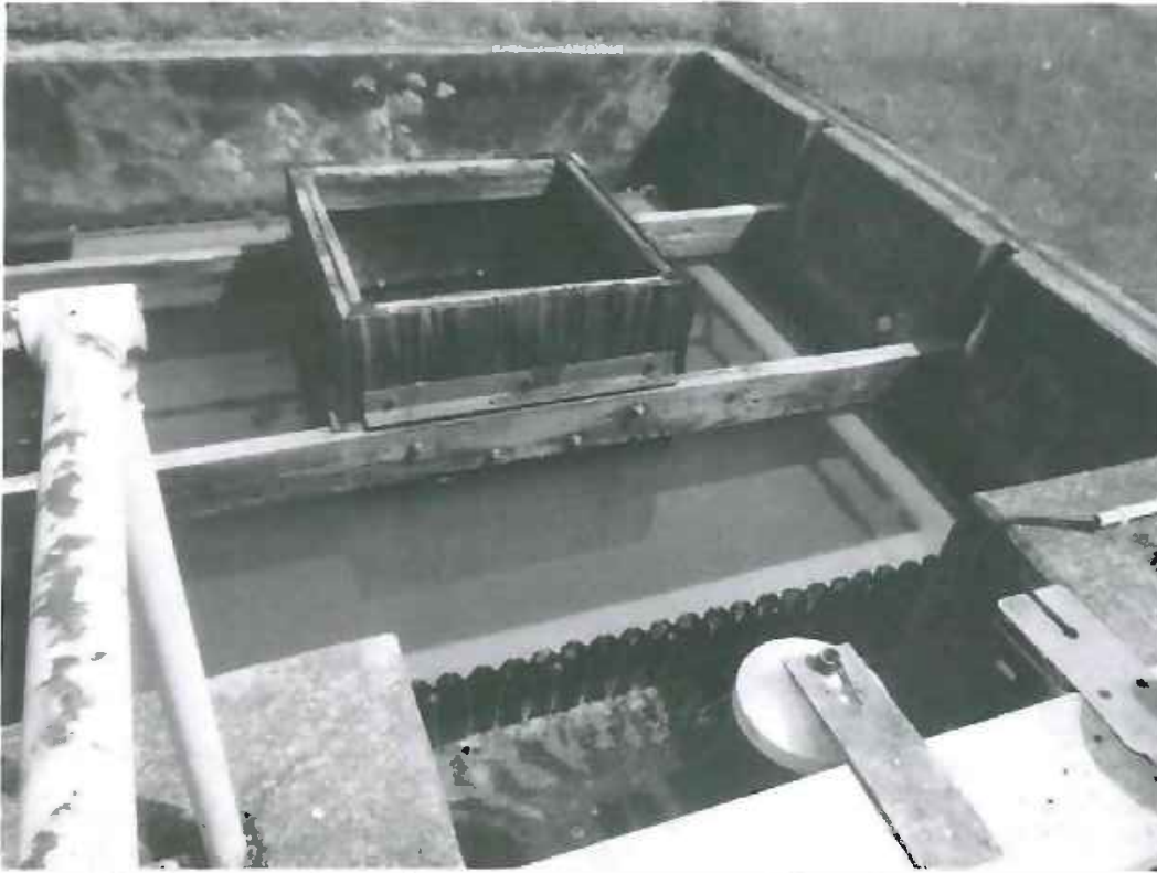
P5070013.JPG – Solids build-up behind weir in final effluent chamber
