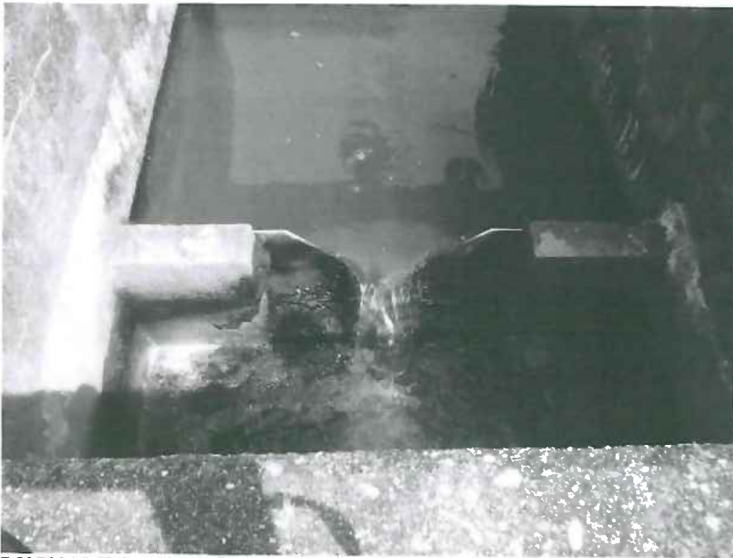
P5070015.JPG – Final effluent and sampling location
