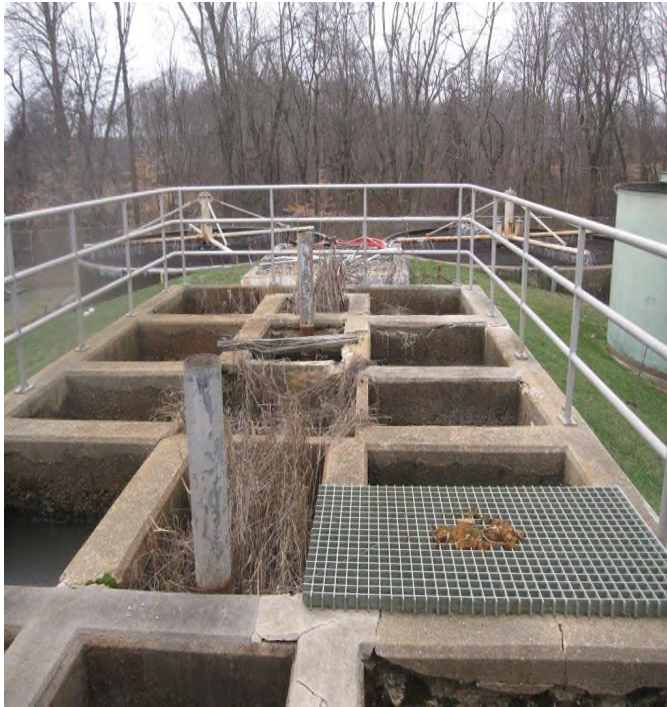
STP Sludge Storage Tank
