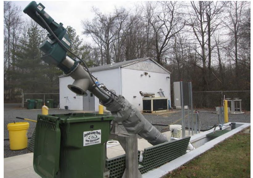
STP Influent Screen (Channel Monster)
