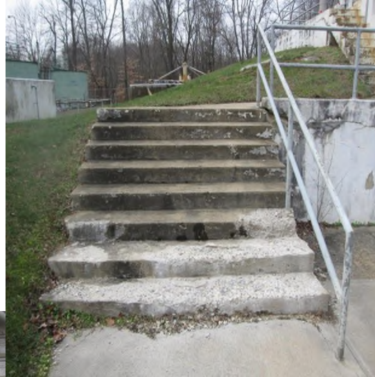
Deteriorated Concrete Steps
