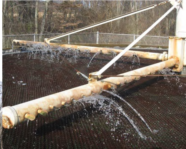
Trickling Filter Distributor Arms
