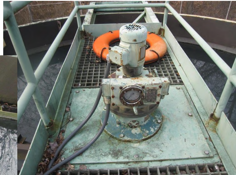
Clarifier Collector Drive
