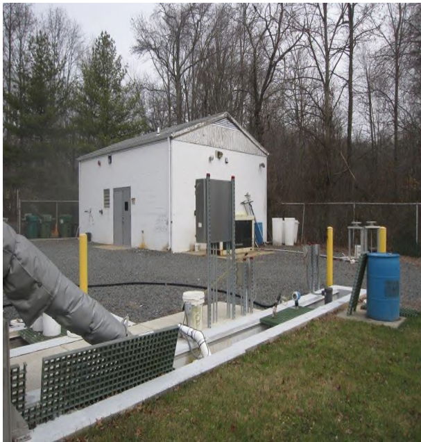
Influent Channel and Flow Meter
