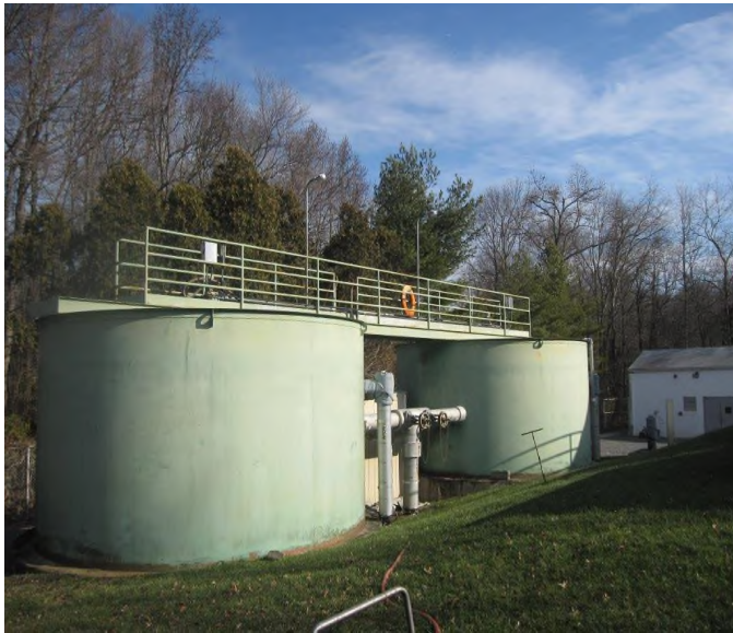
STP Primary Clarifiers
