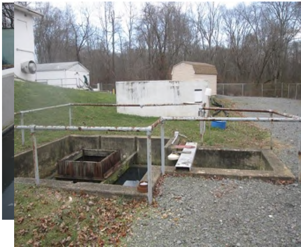
Chlorine Contact Tank
