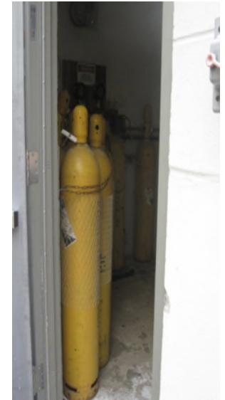
Sulfur Dioxide Cylinders
