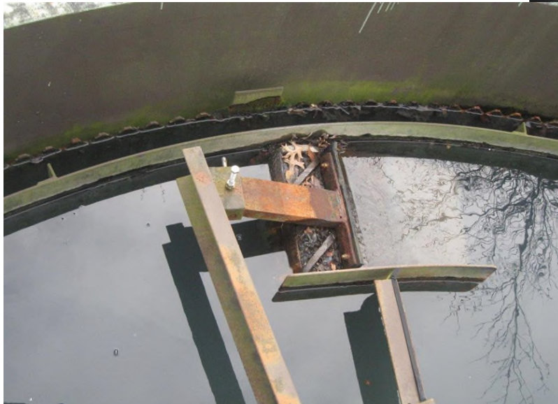
Clarifier Scum Collector
