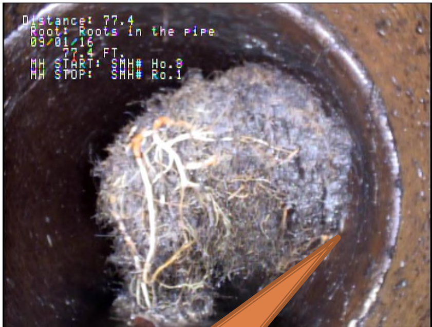
ROOTS ALONG PIPE BARREL
